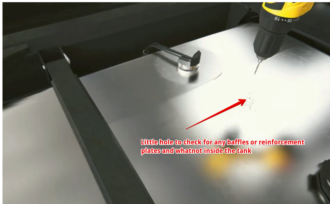
Fig. 31 Drilling a hole to later probe for any obstacles inside with a piece of wire
